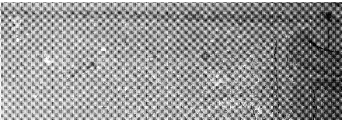
Figure 12: Resulting metal dust at base of rail from gauge wear
