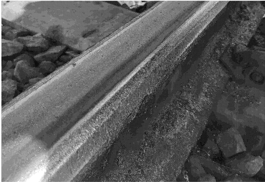
Figure 18: High rail of yard curve showing high degree of metal shavings
