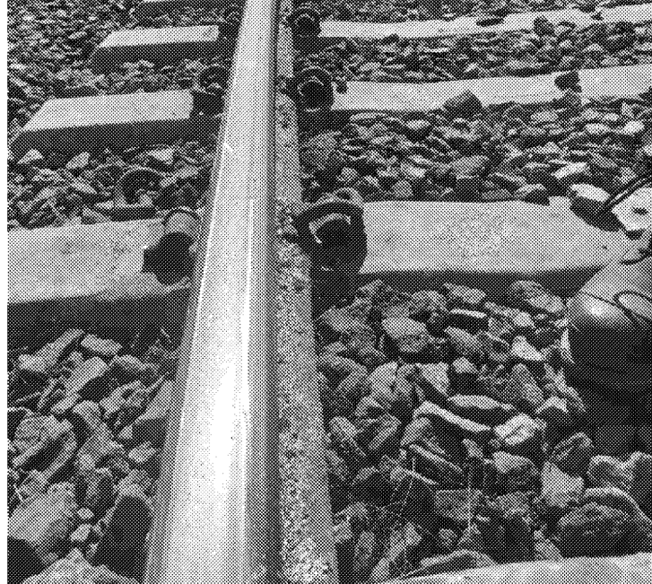
Figure 3. Wheel flange marks on top of rail
