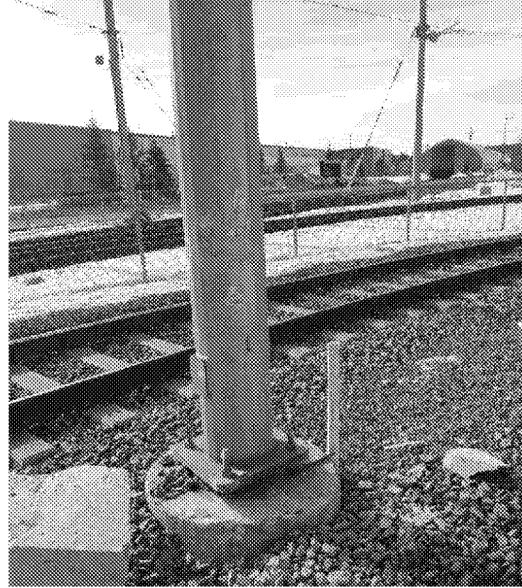
Figure 6. Damage to OCS pole
