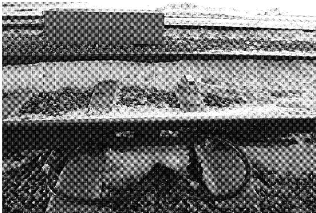
Figure 10: Photo of Buried OCS Rail Bonds at Tremblay
